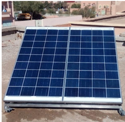
Fig IV. 3. Set up of the test bench on the building roof of the Technical High School in Errachidia city (with a tilt angle of 30^\circ ).
