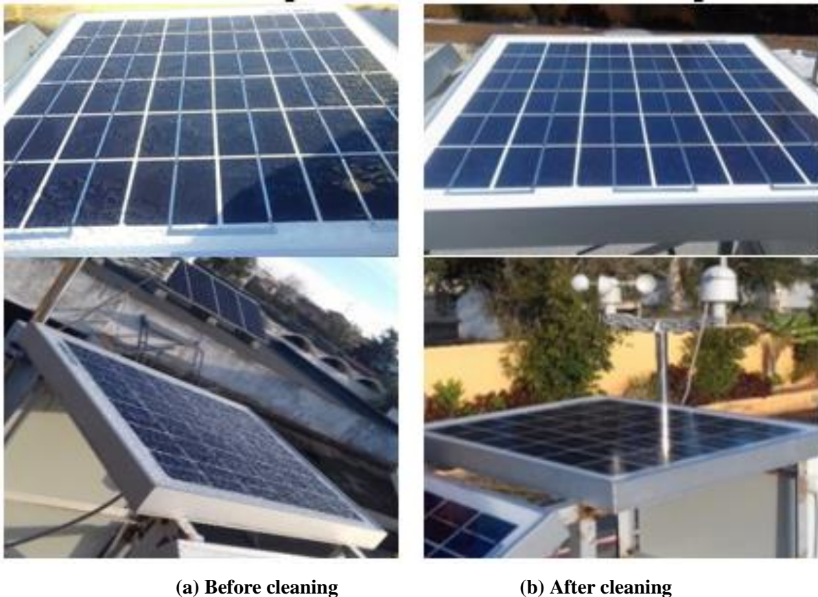
Fig IV. 16. Cleaning tests of small PV modules exposed in RDI Solar Energy Platform of PSES at ENS-Rabat.
