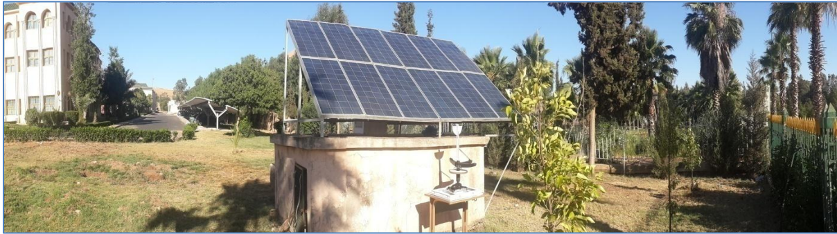
Figure IV.52 : Image of the photovoltaic pumping installation at FST of Settat.
