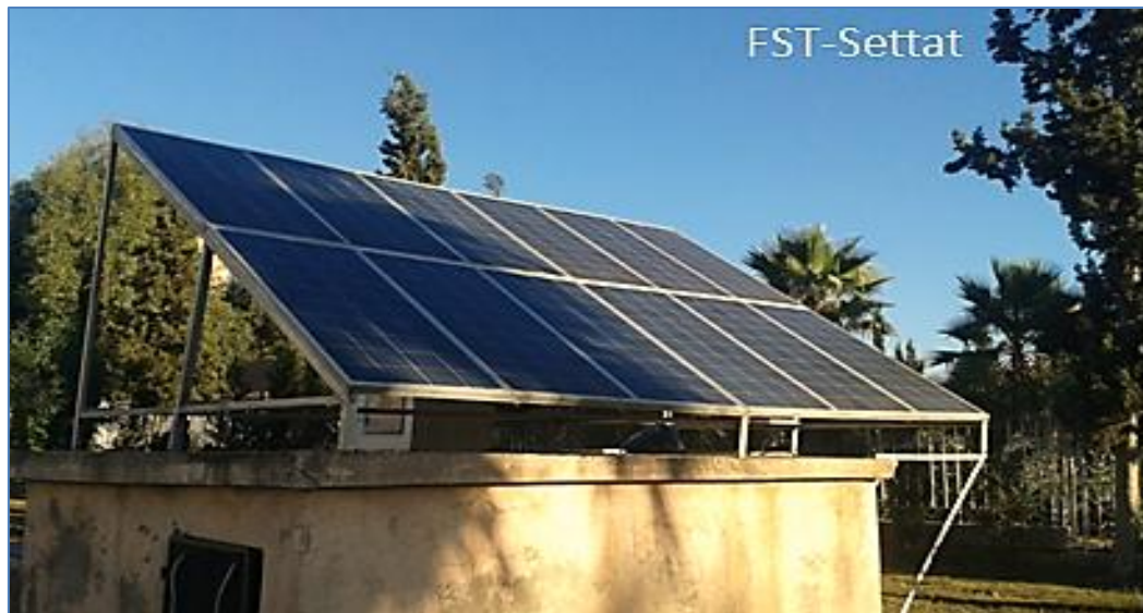
Figure IV.60 : The shading on the our installation at FST Settat.
