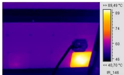
Fig.1.19. Hot spot detected using infrared camera
