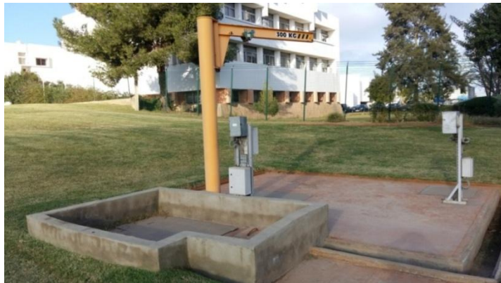
Figure 1.23. Bache de surverse.
