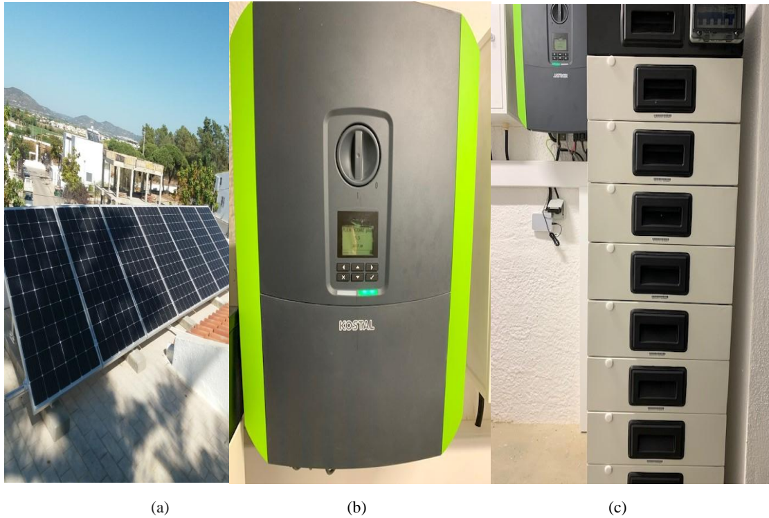
Figure 4-2. Case study house details: (a) photovoltaic panels, (b) inverter, (c) battery.
