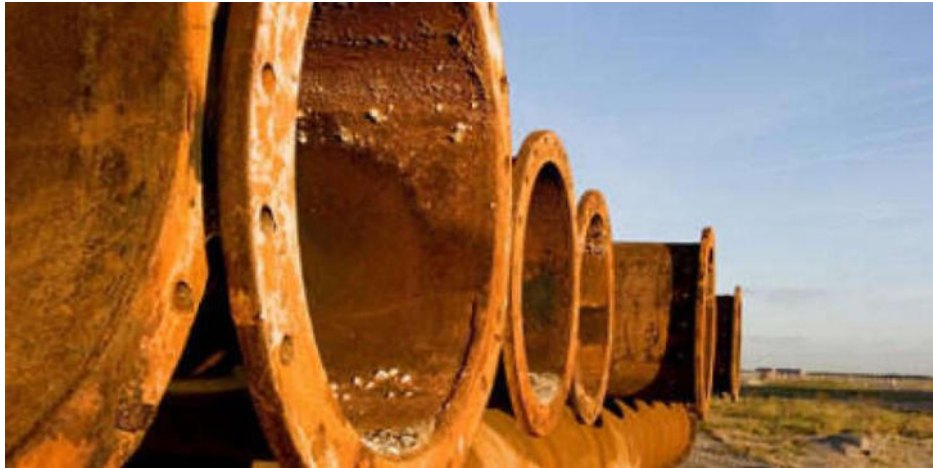
Figure I. 2. Corrosion des tuyaux[38].
