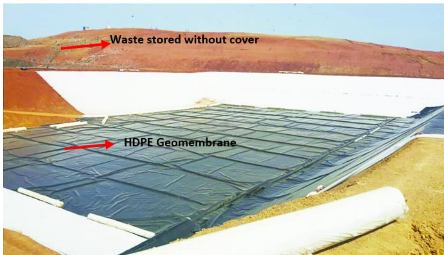
Figure 2-4. The configuration of the lining system of Oum Azza' landfill cells and lagoons.
