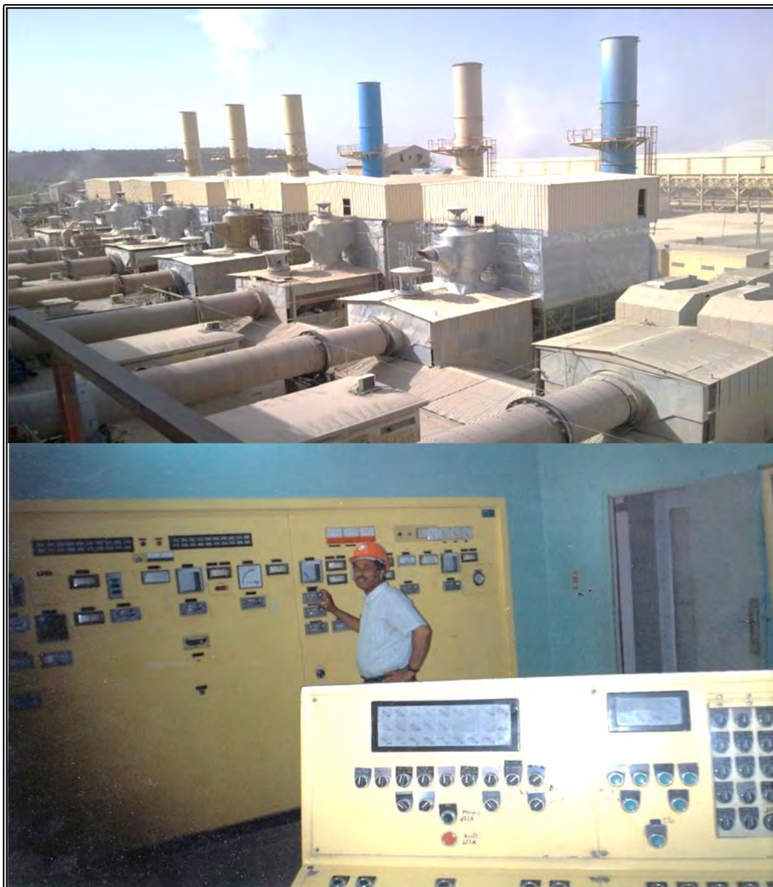
Fig.8: The drying and calcination plant as well as the control room, in Béni-Idir.
