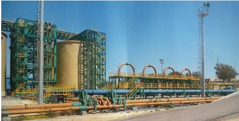
Figure 12: Throttling station (choke station)
