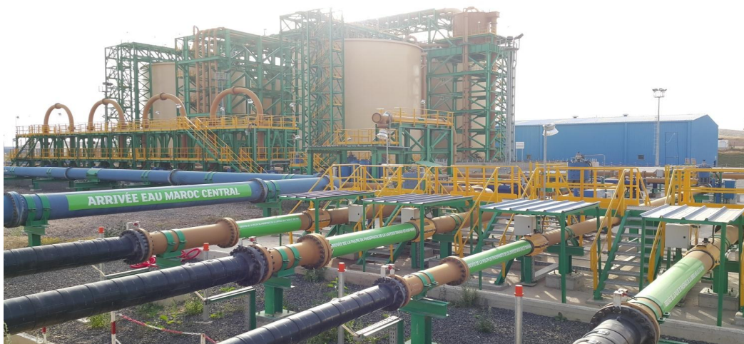
Figure 11: Pipelines from washing plants
