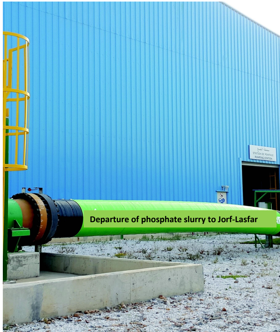
Figure 3: pipeline of transport of the phosphate slurry (Group OCP)
