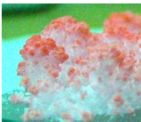
(c) efflorescence chou-fleur
