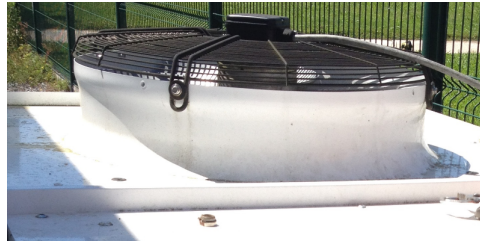
FIGURE 2.26: Cooling tower used in the solar cooling installation
