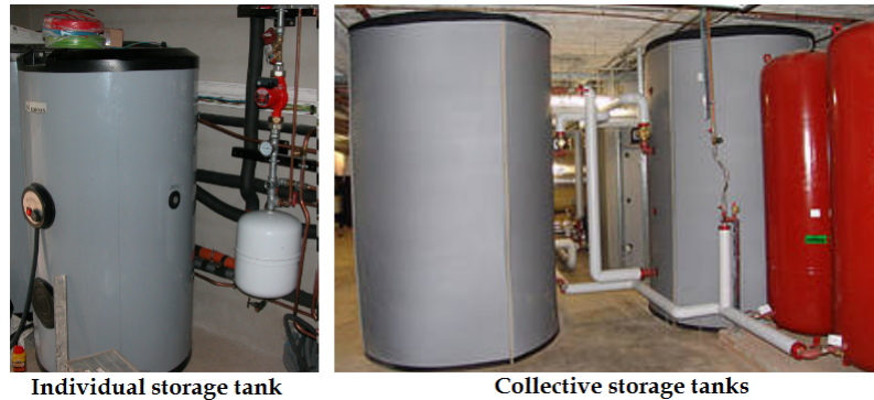
FIGURE 2.3: Example of storage tanks used in solar DHW, heating and cooling systems (Bouhal et al., 2017b)
