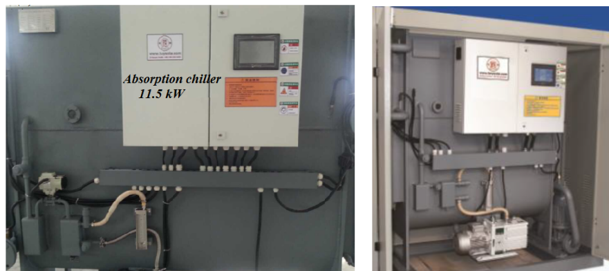
FIGURE 2.25: Solar absorption chiller RXZ-11.5 kW implemented in Ben Guerir ( Green Energy Park )
